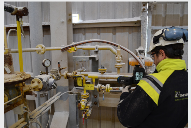
Philip Schraeyen and Jan Van Hout of The Sniffers using the GF77 camera to inspect for methane leaks
